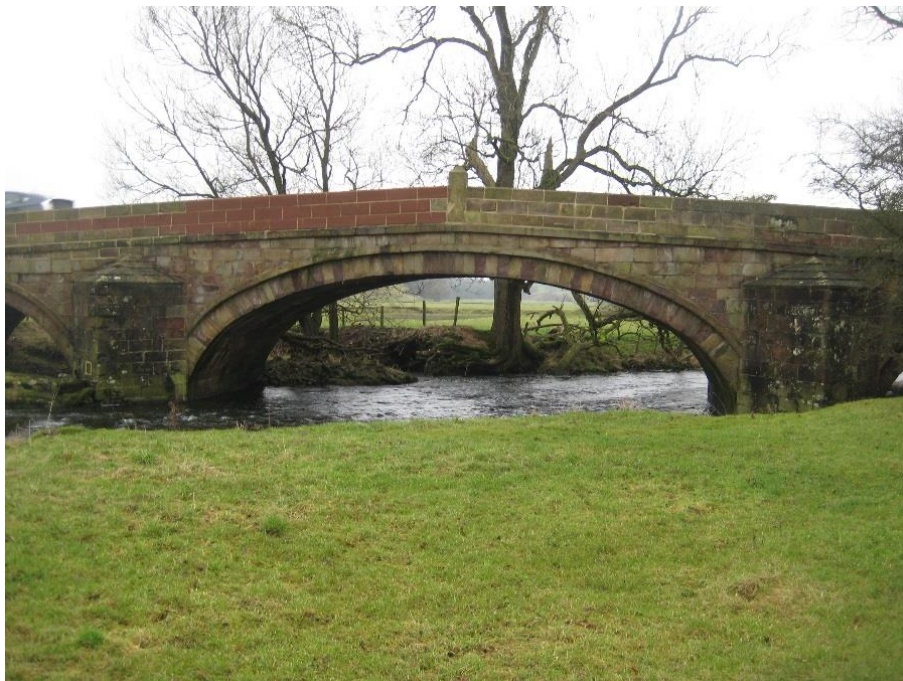
Centre span upstream elevation recent parapet damage which has been repaired with a red stone.
